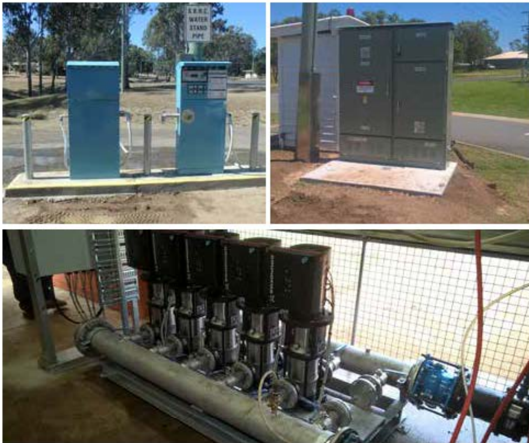
(top left) Water stand pipes upgrade/replacement. (top right) Houghton Street sewer pump station. (Below) new pumps at Retschlag Street.
