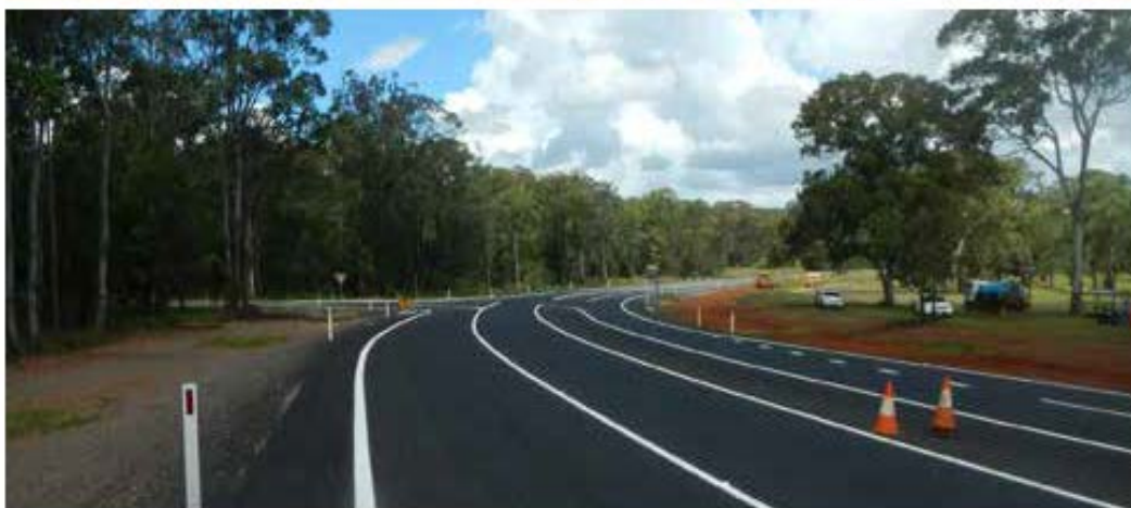
(top left) Gravel Resurfacing at Bullock Runnymede Road, Bullock (top right) New footpath at Rodney Street, Proston (above left) D'Aguilar Highway, Coolabunia Intersection Upgrade, Coolabunia Road and Mary Street.
