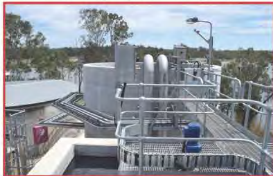
The Gordonbrook Water Treatment Plant [photo courtesy of South Burnett Online]
