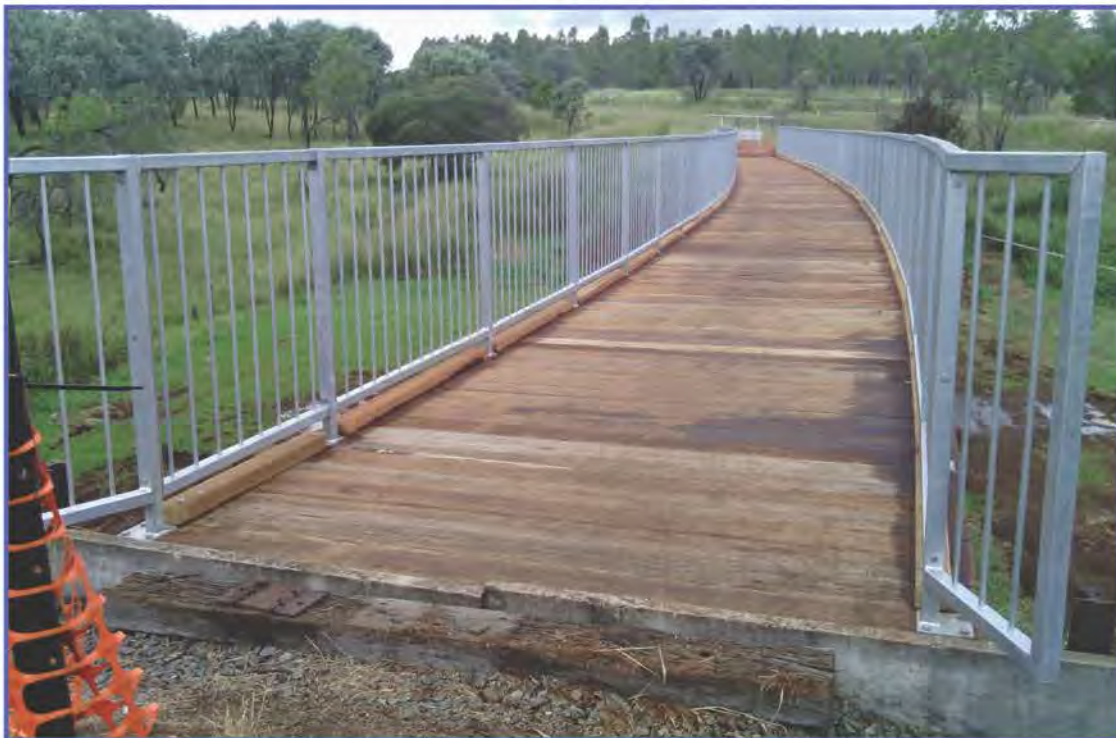
Construction of the Tingoora bridge on the Kilkivan to Kingaroy Rail Trail
