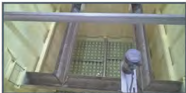
The newly refurbished filter trains at the Murgon Water Treatment Plant
