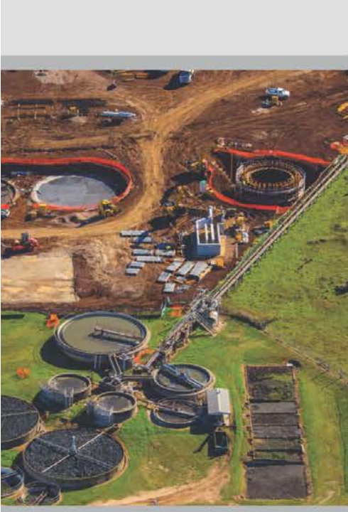
Above: Progress of construction work at the new Kingaroy Wastewater Treatment Plant in April 2014. The existing Kingaroy Wastewater Treatment Plant in the foreground.
