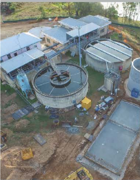
Above: Progress of the upgrade works at Gordonbrook Water Treatment Plant – June 2015
