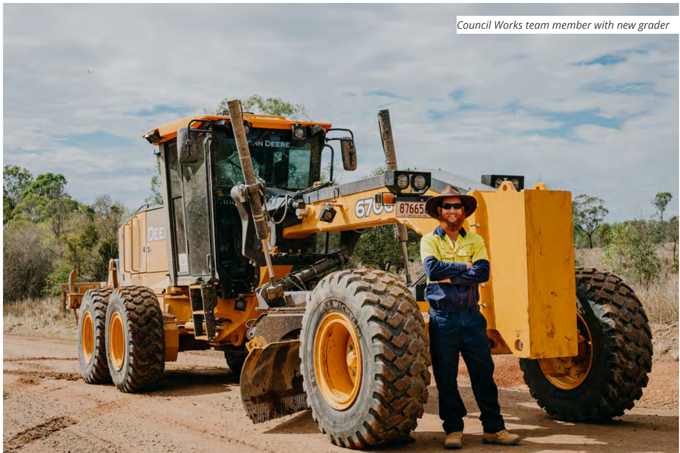
Maidenwell Bunya Mountains Rd - Upgrade to sealed standard and realignment at Wengenville Glenclyffe Rd
