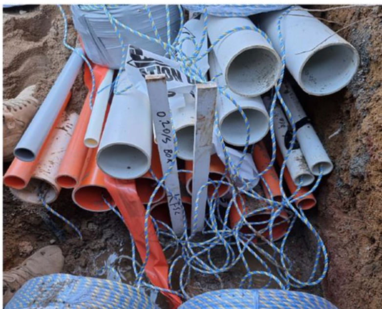
Image of Conduit Bundle – north side of Alford St – showing complexity of buried services
