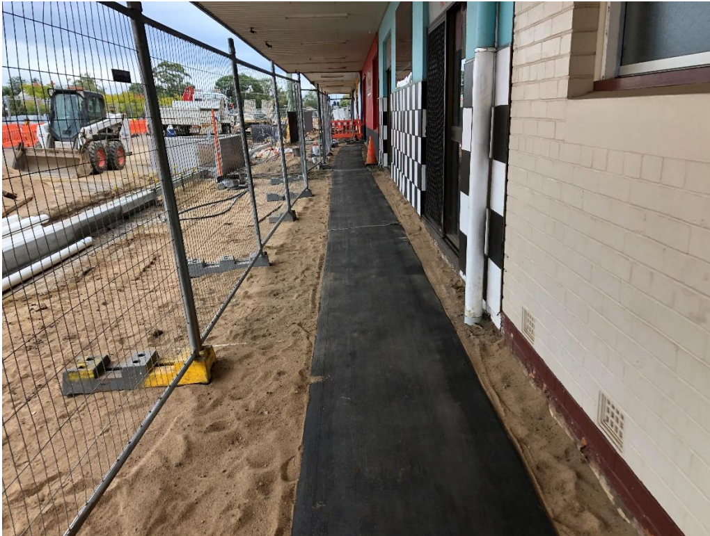
Image of footpath north side of Alford Street showing temporary footpath for shop access
