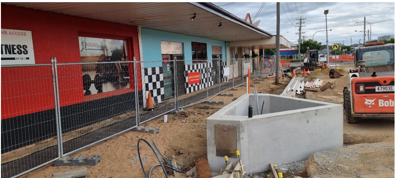
Image of first raised planter poured, also showing temporary footpath in background.
