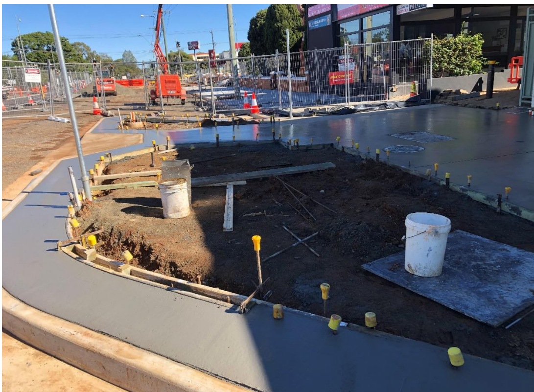
Image of garden bed at Asian Gourmet with freshly laid concrete maintenance strip.
