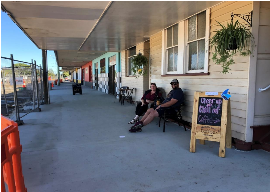
Image of footpath north side of Alford Street partially complete with local residents enjoying a Saturday coffee in the new on street dining area at Hunter Gatherer Trader
