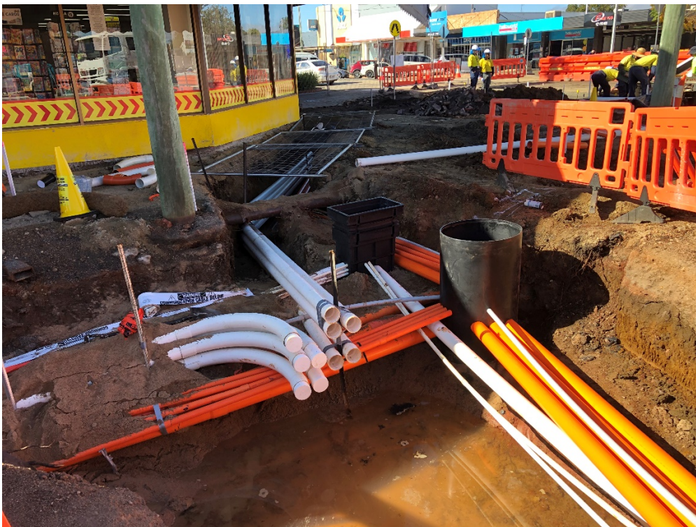
Image of web of conduits installed by contractors and Council teams at Glendon / Alford Streets.
