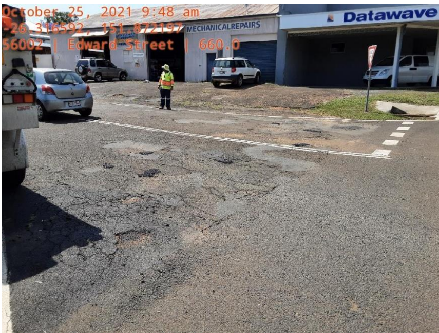
Edward Street, Wondai pot hole repairs, this street is being proposed for LRCI 3 funding.
