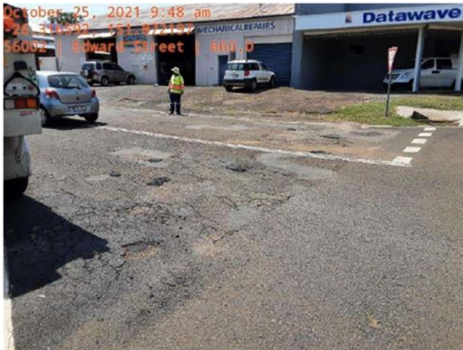
Edward Street, Wondai pot hole repairs, this street is being proposed for LRCI 3 funding.
