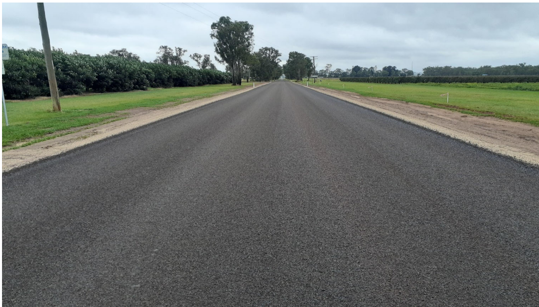
Figure 2- Kumbia Road - Road widening and reconstruction project from chainage 19.1km to 19.8km
