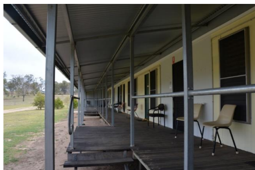
Figure 243. View facing south-west along the front verandah of the accommodation building, providing access to the individual bedrooms, kitchenette and bathroom.
