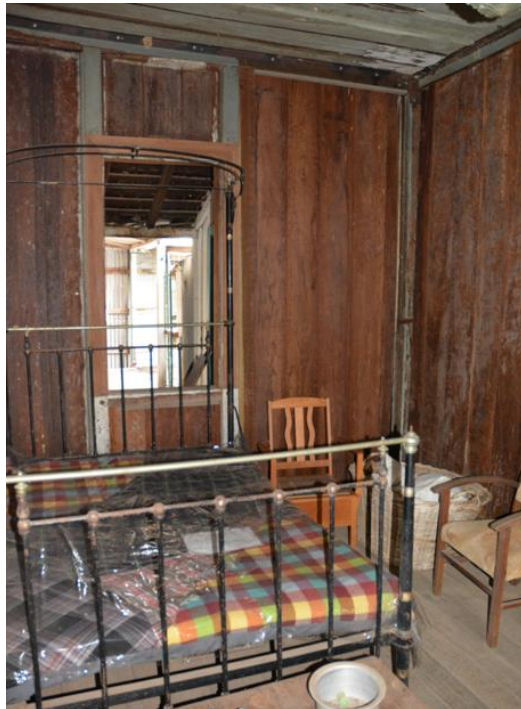
Figure 114. Interior of Bedroom 2. Note the sash window opening onto the rear verandah.
