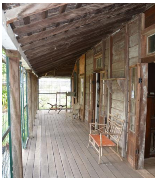
Figure 91. View along the front verandah of the main homestead, showing the eastern end of the verandah.
