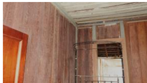
Figure 113. The south-east corner of Bedroom 2, which is showing evidence of water penetration affecting the timber ceiling fabric.
