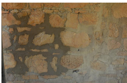
Figure 139. Detail of a section of re-pointed stonework utilising the incorrect mortar mix, as part of previous restoration works.
