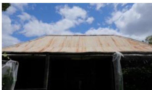
Figure 85. The north-east (front) elevation of the main homestead, showing the long-ridge hipped roof, clad in corrugated galvanised iron.
