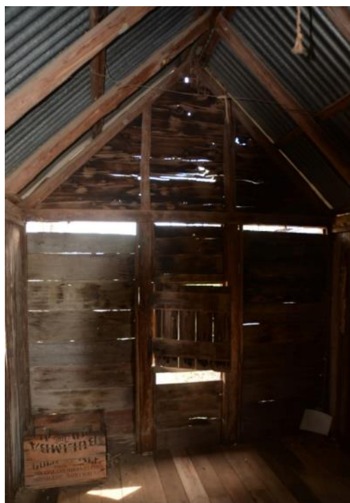
Figure 174. Interior of the postal receiving office with the timber casement window visible in the centre.
