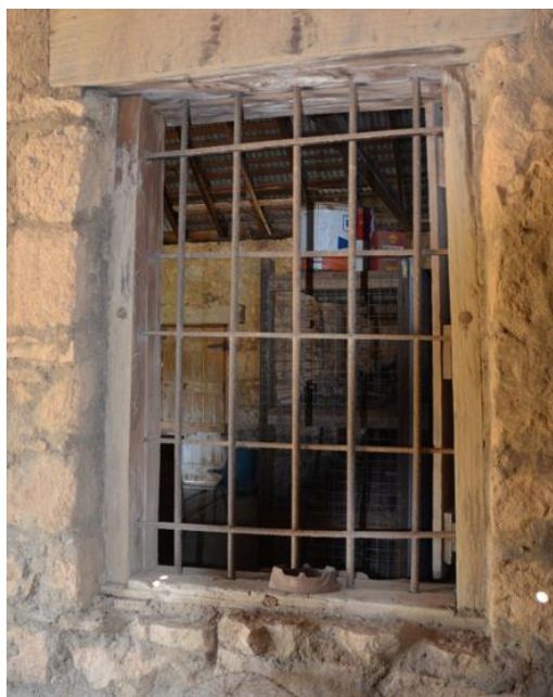
Figure 149. Detail of a typical window with timber lintels and frames and iron bars.
