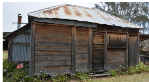
Figure 202. The north-east elevation of Brownie's hut. Note the wide timber weatherboard slabs, fitted horizontally.
