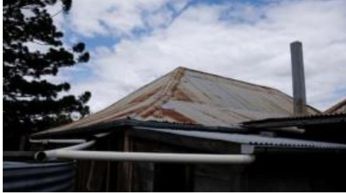
Figure 86. View facing north-east showing the 'broken back' roof profile of the main homestead, and the skillion-roof of one of the small extensions.
