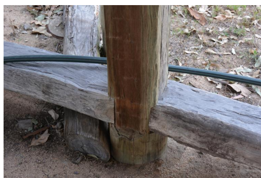
Figure 162. Detail of the intersection of a column and bearer reconstructed using traditional bush carpentry techniques.
