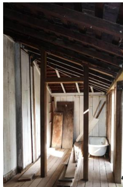
Figure 97. View along the rear enclosed verandah area on the homestead's south-west elevation.
