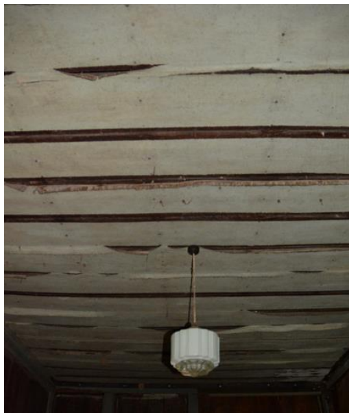
Figure 116. Detail of the dilapidated calico ceiling lining in Bedroom 2.
