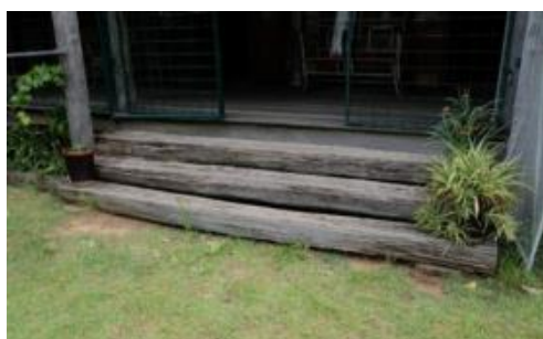
Figure 84. The timber entrance steps providing access to the front verandah of the homestead.
