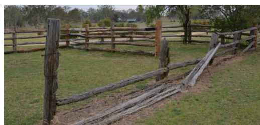
Figure 182. View facing south-west from showing the combination of dilapidated timber posts and rails comprising the former stockyards and recently reinstated erect sections.
