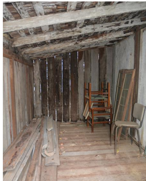
Figure 111. Interior of the addition to the eastern wall of Bedroom 1, which is considered to be a former nursery area.
