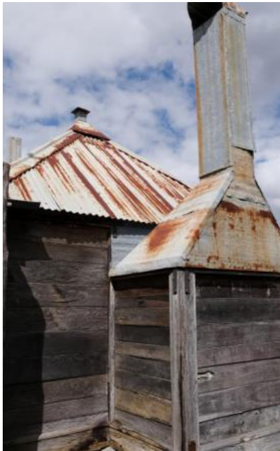
Figure 94. Rear of the detached kitchen on the south-west elevation of the main homestead, showing the pyramid roof profile and galvanised metal-clad chimney.
