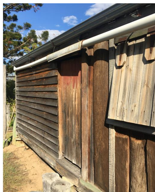
Figure 93. Detail of the external wall of the homestead's north-west elevation, illustrating the use of a variety of materials including unpainted weatherboards, fixed horizontally, and wide chamber boards, fitted vertically.
