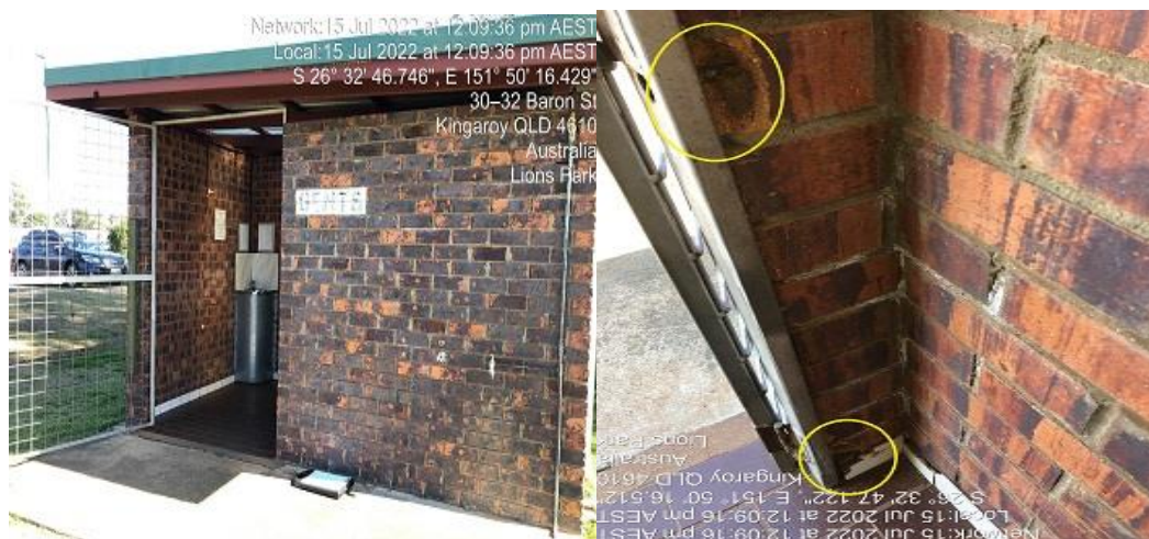
Gates swing out and cannot be secured
