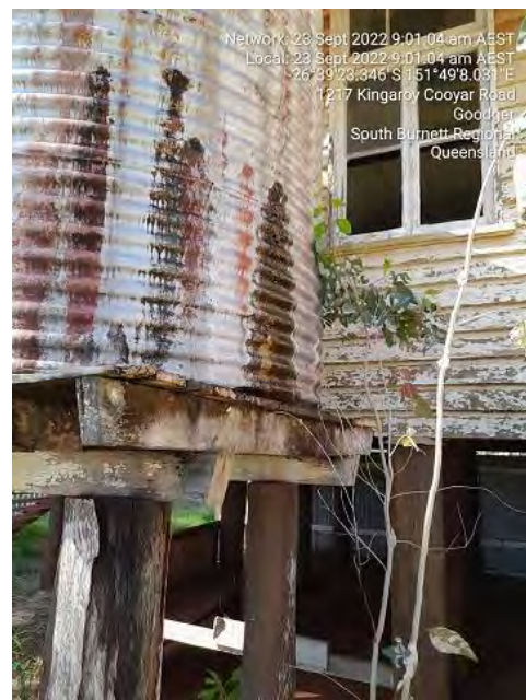
Rotted tank stand.
