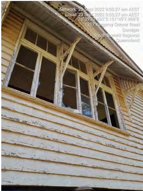
Typical damaged windows
