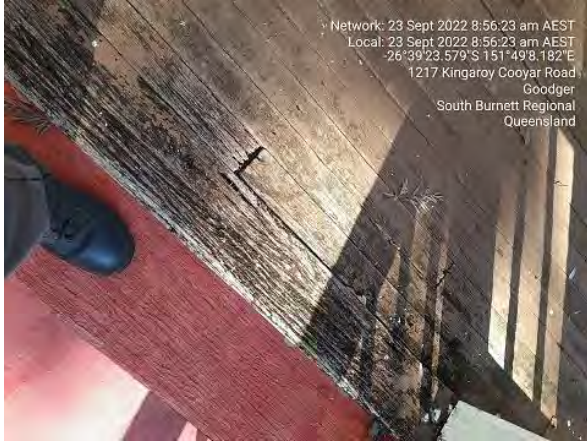
Deteriorated decking boards.
