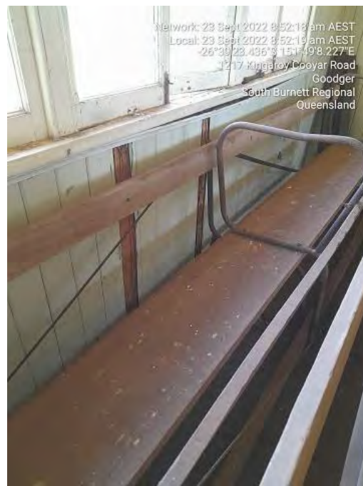
Internal termite damage.
