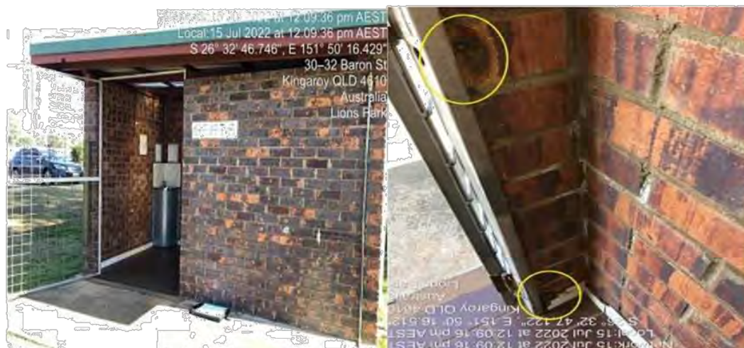
Gates swing out and cannot be secured
