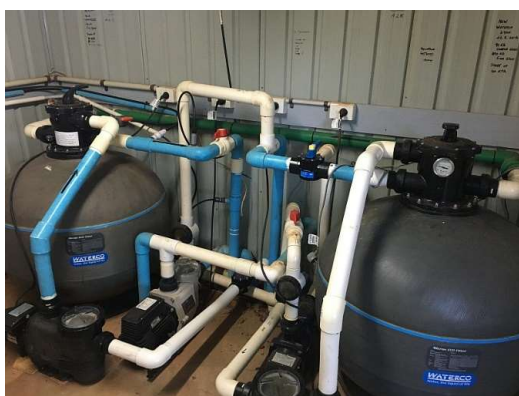
Existing Pool Filters.
