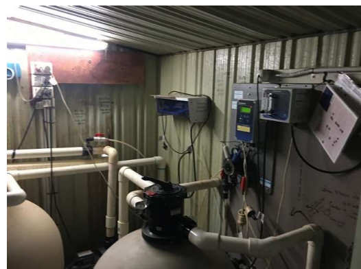
Learn to Swim Pool water treatment plant.
