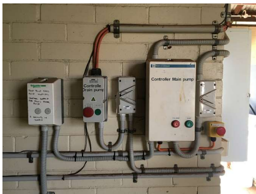
Existing Pool Electrical Controls.
