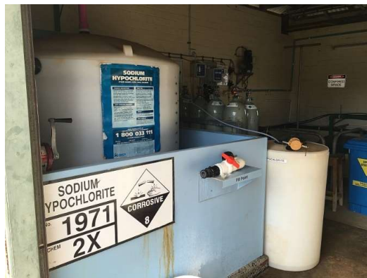
Sodium Hypochlorite Storage Tank and Bund.
