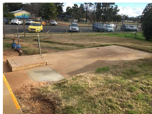
Non-Compliant Truck Loading.
