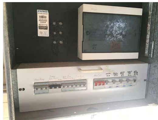
Compliant Circuit Breakers.
