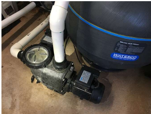
1 of 2 Pool Filter Pump.
