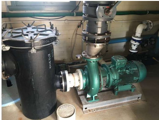
Pool Filter Pump.
