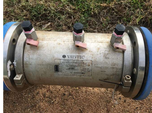
Double Check Valve Backflow Prevention Device.
