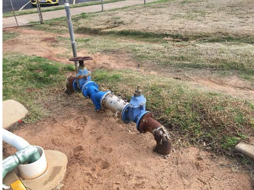
Incoming Water Supply.
