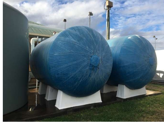
Rear of Filters.
