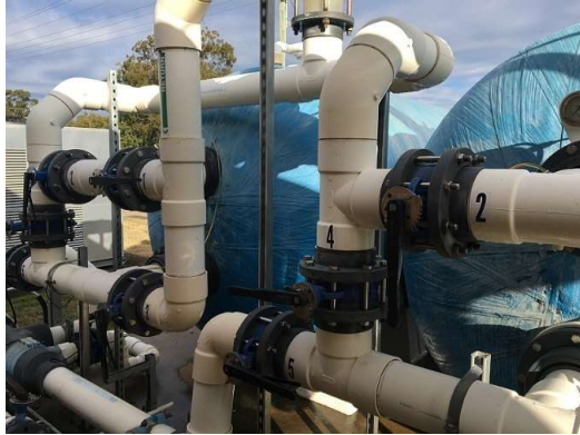
Existing Pool Filter Face Plumbing.
