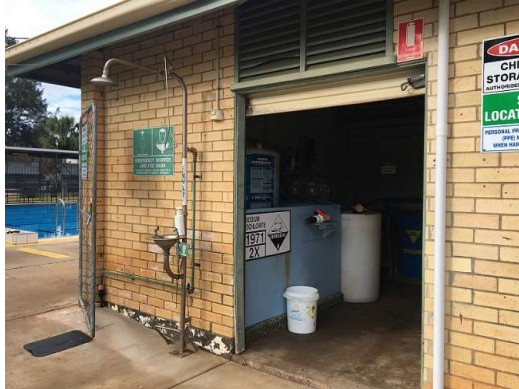
Existing Safety Shower <2m from Tank Fill Point.
