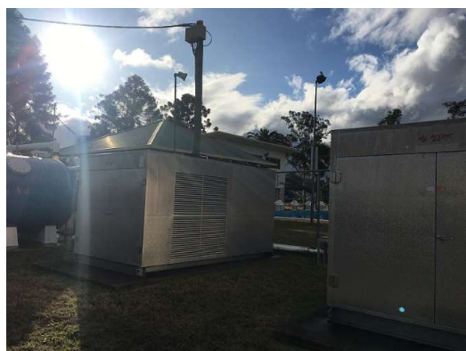
50m Pool Heat pumps.
