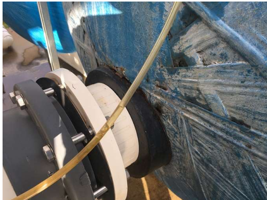
Signs of Surface Delamination.
