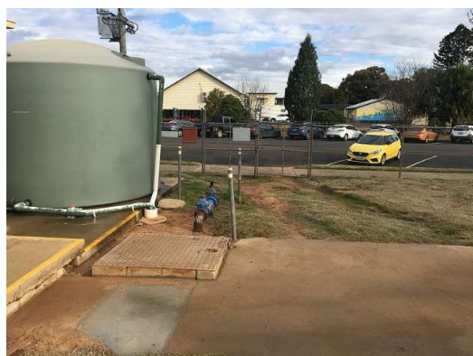
Existing Backwash Tank.
