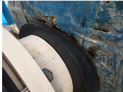
Inlet and Outlet Pipe Degradation.
