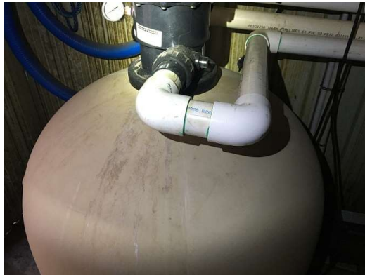
Existing Pool Filter 1 of 2.
