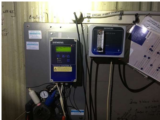
Pool Water Chemistry Instrument (left).
