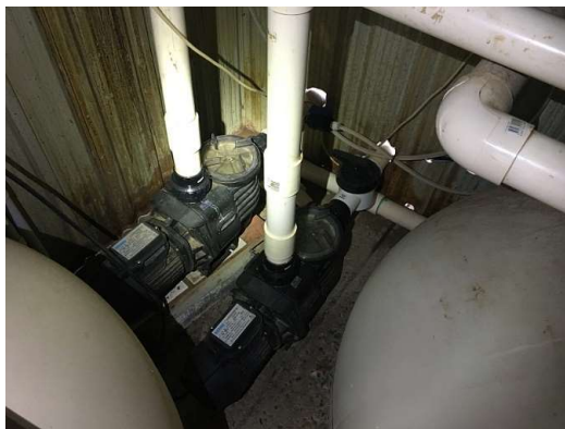
Pool Filter Pumps.
