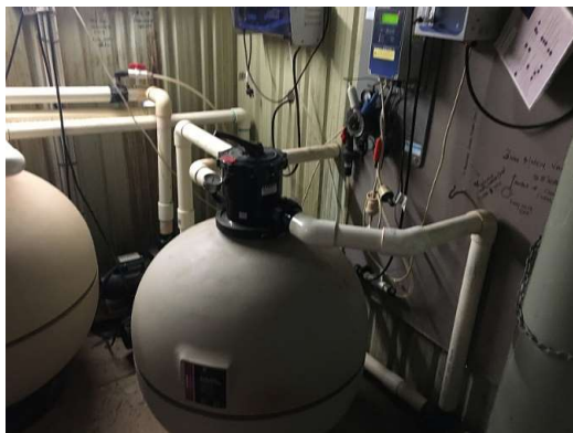
Existing Pool Filter 2 of 2.
