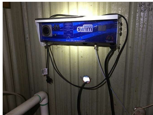
Salt Chlorinator Controller.
