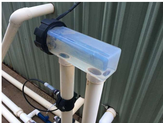
Existing Disconnected Salt Chlorinator Cell.
