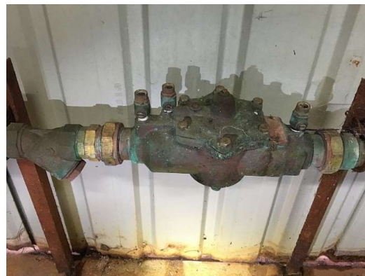
Backflow Prevention Device.
