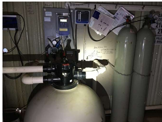
Pool Water Chemistry Dosing.
