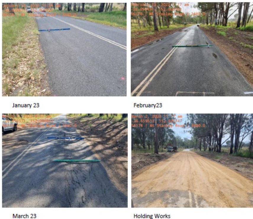
Photo: Mt Stanley Road - Nanango – REPA Scope Creep over 2 Months & Holding Works.
