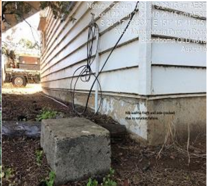
Nib wall cracked.
