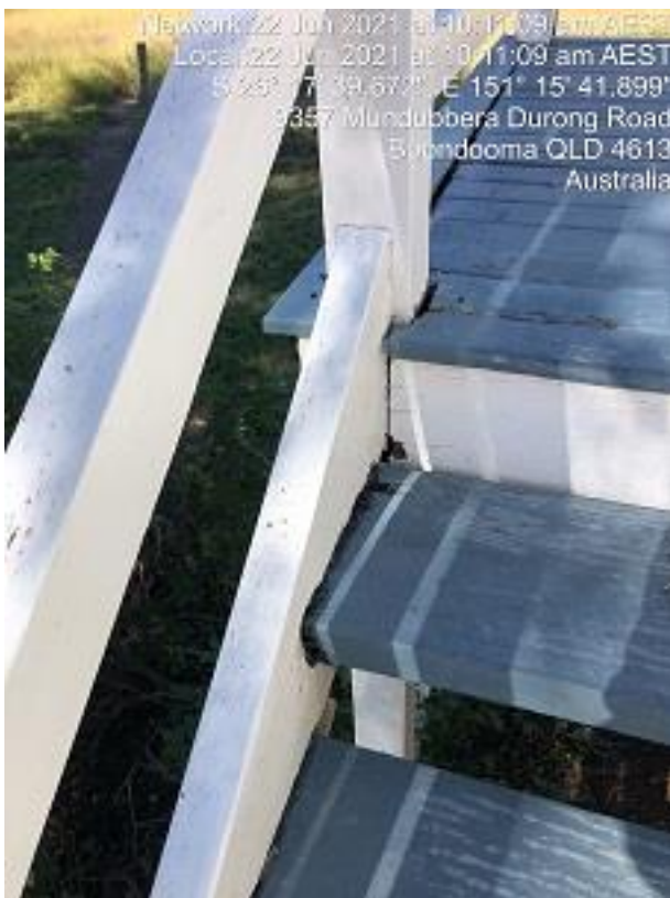
Deteriorated rear stairs.
