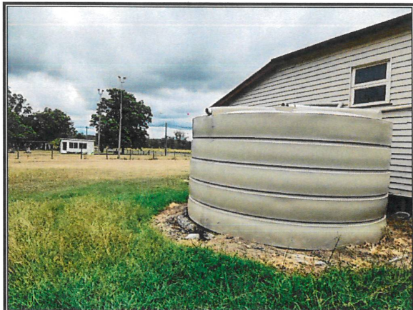
Tank overflow discharging to ground surface with the tank leaning back towards the hall
