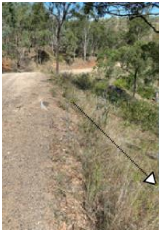
Figure 3: Steep batter from edge of formation
