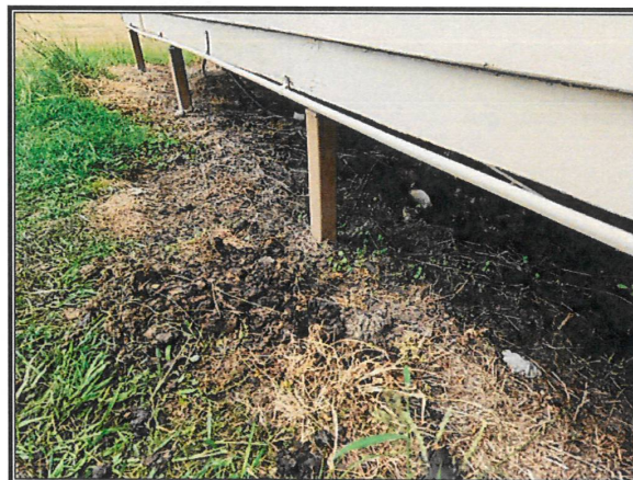
Ponding of water evident in subfloor (south eastern corner of hall)
