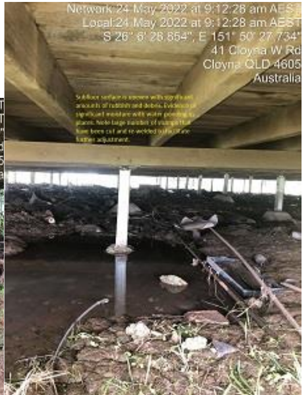
Water laying under building.
