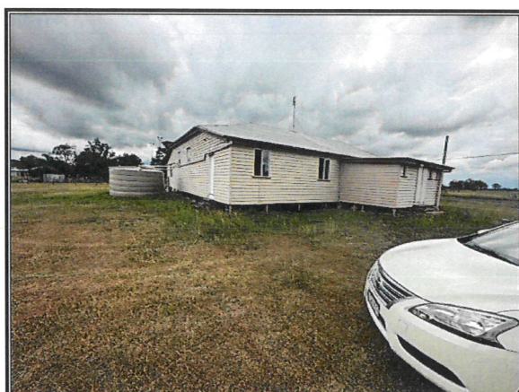
Poor site drainage to eastern and southern sides of hall
