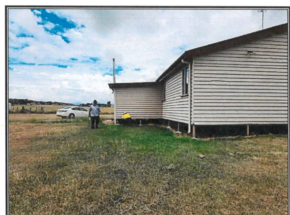
Poor sit drainage to eastern side of hall
