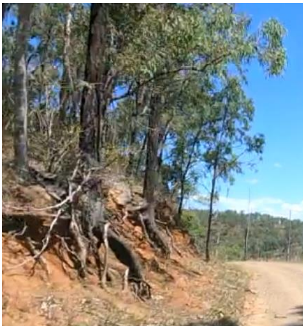
Figure 4: Batter on inside of substandard curve
