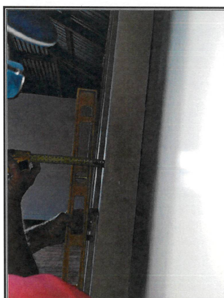
Lean of internal stud wall. Approximately 30mm in 1000mm. Total of 107mm over full height of wall.
