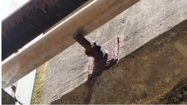
Figure E: Telecommunication conduit resting on a transverse stressing bar, increasing oxidization of the bar, and preventing the road authority from undertaking maintenance (replacement of the bar). This bar is critical to bridge integrity and safety.
