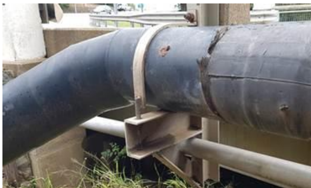
Figure D: Telecommunications conduit installed through a water pipeline bracket.
