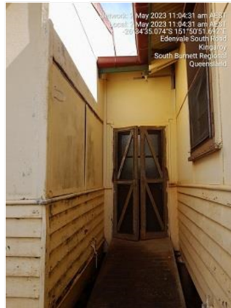
Cladding and paint in poor condition.
