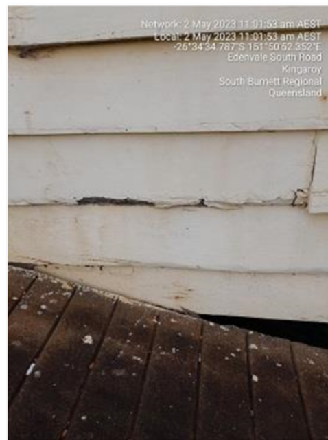
Typical rot to weatherboards.
