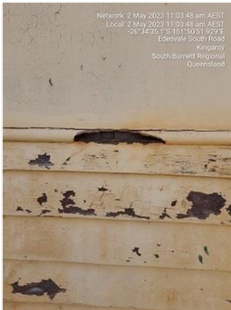
Cover strip and paint in poor condition.
