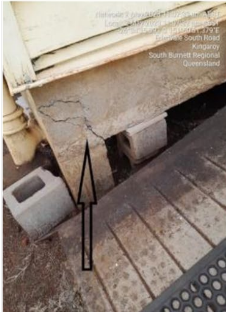
Cracked slab-note concrete block support.
