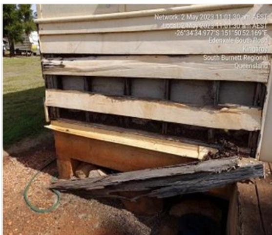
Termite damaged to weatherboards.
