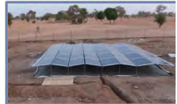
Kalom, Senegal, 20kWp (2016)
