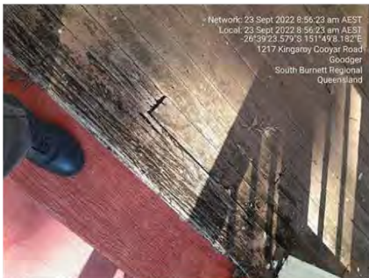
Deteriorated decking boards.
