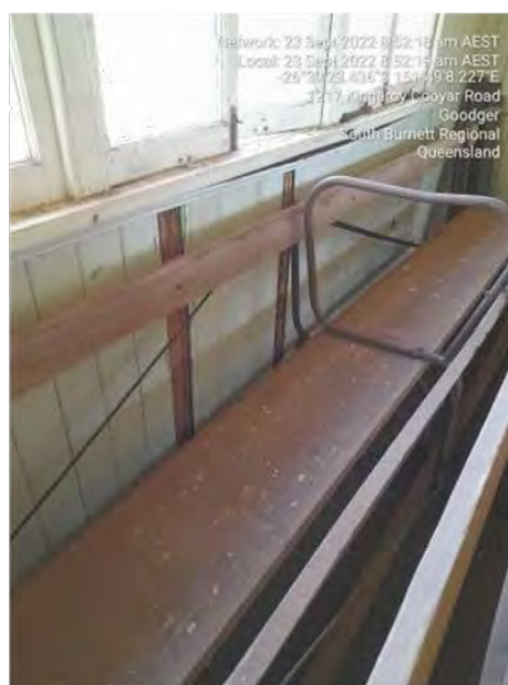
Internal termite damage.
