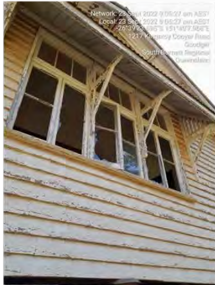
Typical damaged windows
