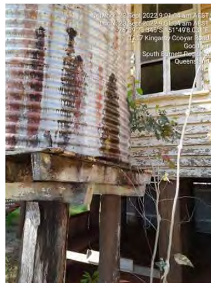
Rotted tank stand.
