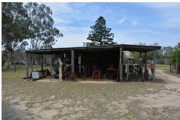
Figure 179. The south-west elevation of the machinery display shelter. Note the timber partitions dividing the shelter into separate sections.
