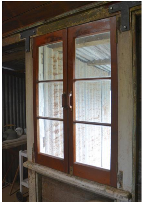
Figure 125. Example of the replacement timber casement windows in the kitchen, which are non-sympathetic additions.
