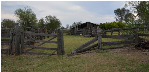
Figure 183. View facing south-west showing the dilapidated section of the stockyards and the milking bails structure behind.
