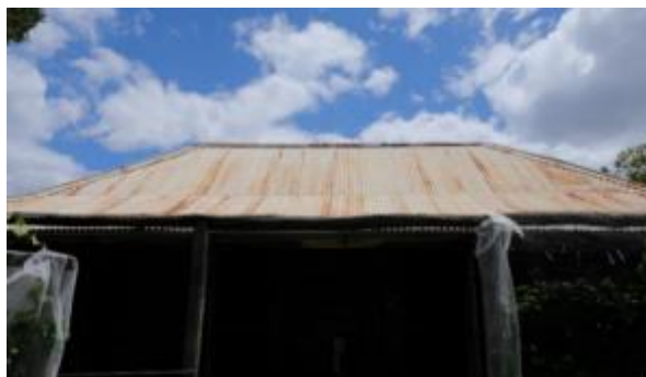
Figure 85. The north-east (front) elevation of the main homestead, showing the long-ridge hipped roof, clad in corrugated galvanised iron.
