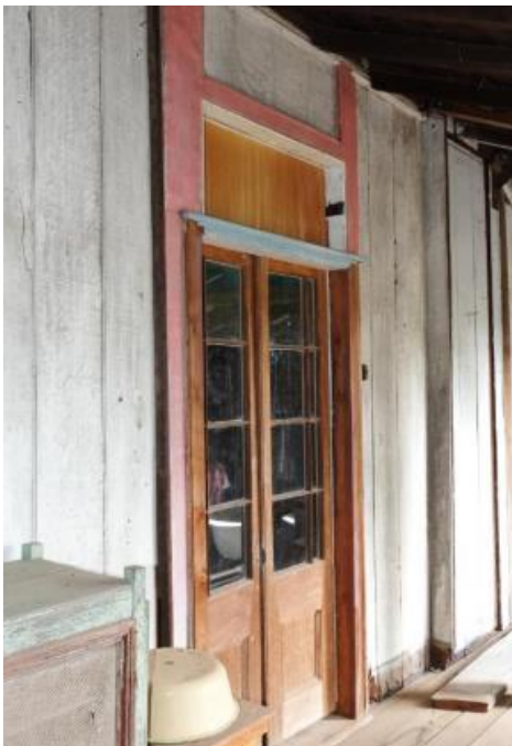
Figure 96. Example of the timber French doors leading from the main bedroom onto the rear verandah, noting the infilled fanlight.
