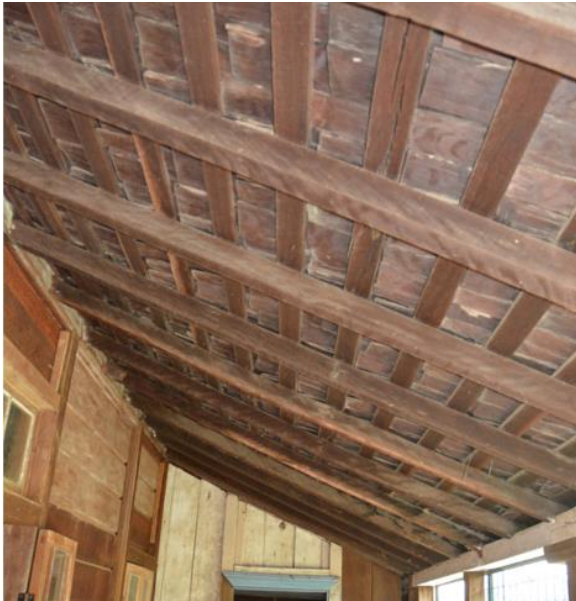
Figure 90. The underside of a section of the front verandah roof, showing the early timber shingles.
