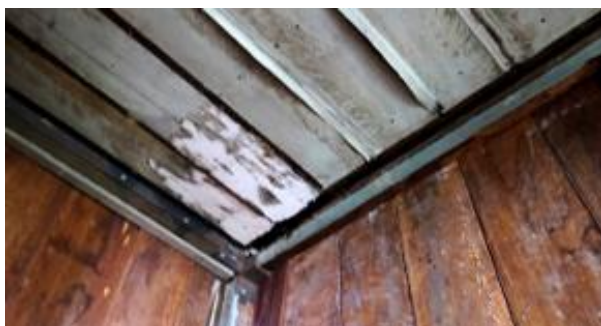
Figure 112. Detail of the north-west corner of the ceiling in Bedroom 2, showing water penetration affecting the ceiling, and movement at wall and ceiling junction.
