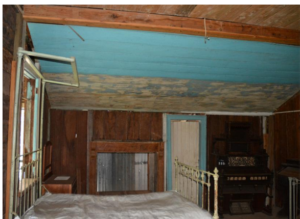
Figure 110. Interior of Bedroom 1 showing the wall under the low side of the ceiling with a small timber slab door that accesses an additional room, which is considered to have been used as a nursery.
