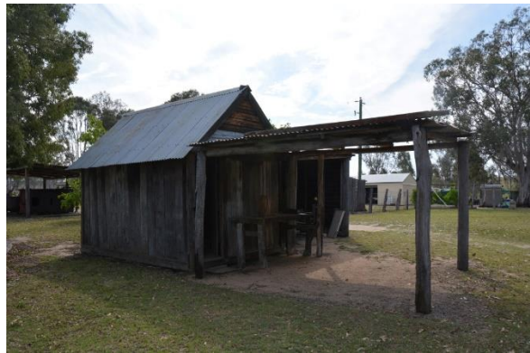
Figure 172. The south-east elevation of the postal receiving office, showing the c.1950s skillion awning attached to the front.
