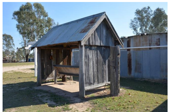
Figure 206. The south-west elevation of the DPI shelter, showing the remnant timber post of the cattle dip installed herein 2006 known as 'Stockie's Stump'.
