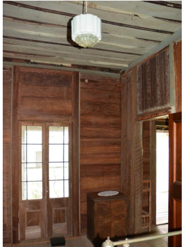
Figure 115. Interior of Bedroom 2. Note the French door opening to the front verandah and the dilapidation of the calico ceiling lining.
