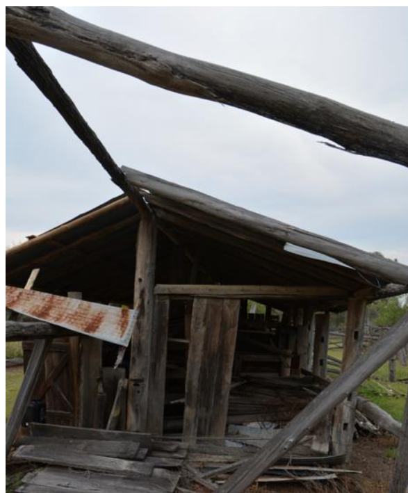
Figure 188. The north-eastern end of the milking bails structure, which is substantially deteriorated.
