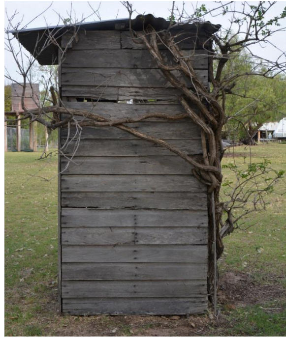
Figure 170. The north-west elevation of the outhouse, showing the extent of the tree growth around the structure.
