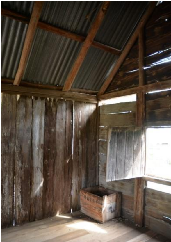
Figure 173. Interior of the postal receiving office, showing the timber slab case window in the rear elevation.
