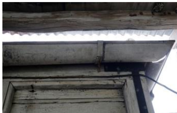
Figure 99. Detail of the half round gutters surviving attached to the northern wall of the homestead's detached kitchen.
