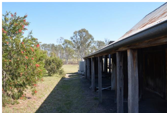
Figure 138. View facing north-west along one of the lean-to verandah additions to the stone store.
