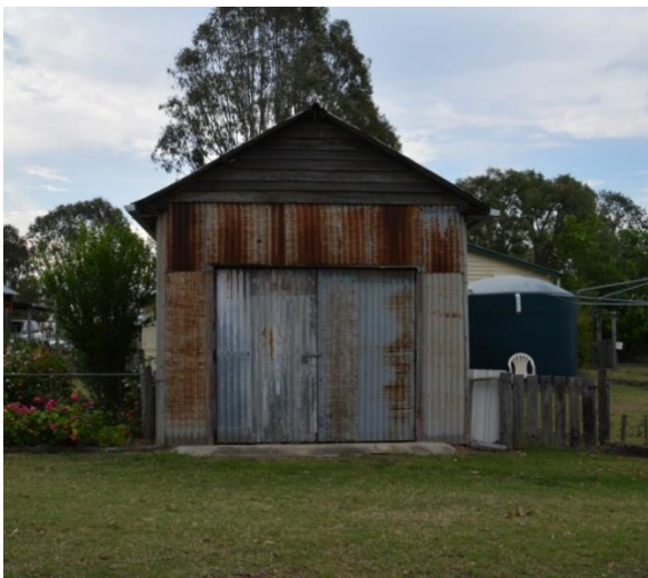
Figure 197. The south-east elevation of the caretaker's store, showing the double door access.
