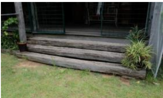
Figure 84. The timber entrance steps providing access to the front verandah of the homestead.
