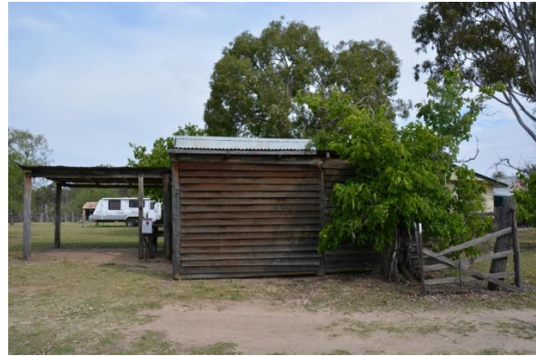
Figure 176. The north-west elevation of the postal receiving office, showing the thin chamferboards used in the c.1950s construction of the carport extension.
