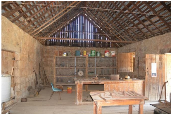
Figure 141. Interior of the north-west end of the stone store. Note the exposed timber rafters and roof framing.
