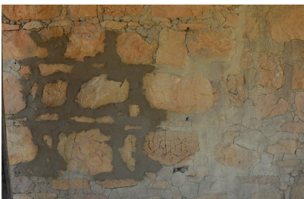
Figure 139. Detail of a section of re-pointed stonework utilising the incorrect mortar mix, as part of previous restoration works.
