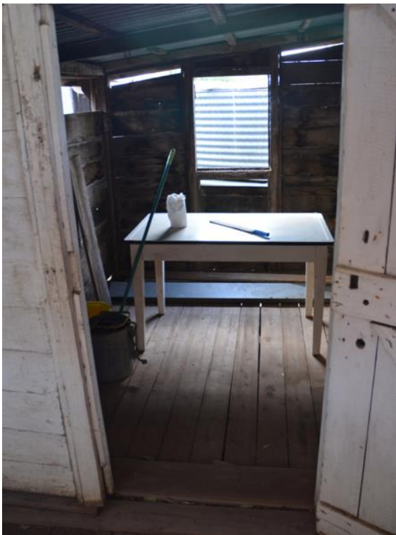
Figure 120. Interior of the small room of unknown use created through the addition of a skillion-roof extension.
