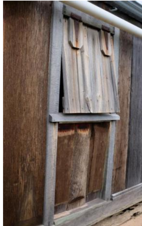
Figure 95. Example of the reconstructed timber window awnings fitted to window openings on the homestead's north-west elevation.
