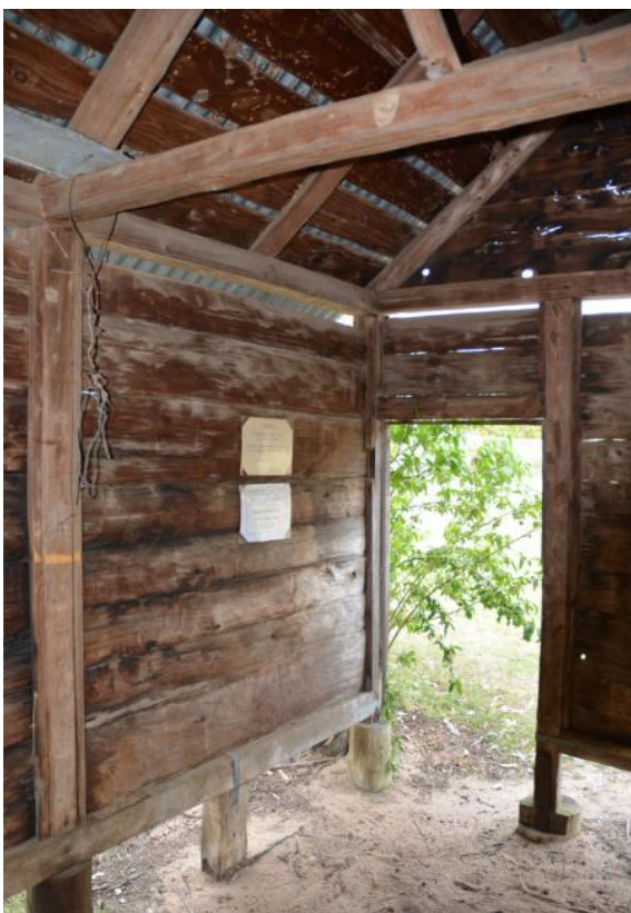
Figure 167. Interior of the cool house, illustrating its construction of horizontal timber slabs of Cypress pine.
