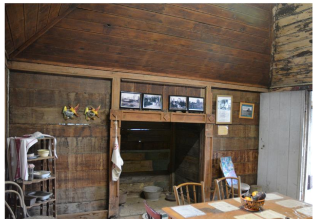
Figure 123. Interior of the detached kitchen, showing the fireplace recess with simple timber mouldings fixed at the joints with the framing.
