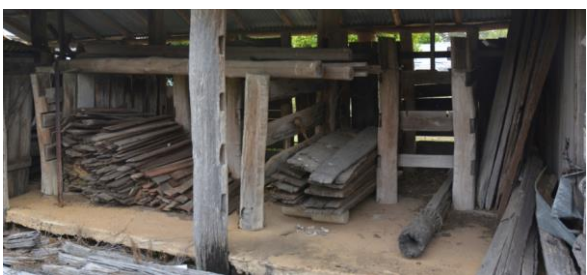
Figure 187. Typical interior view of the milking bails structure, which is not readily accessible due to the use of the structure for storage of timber.
