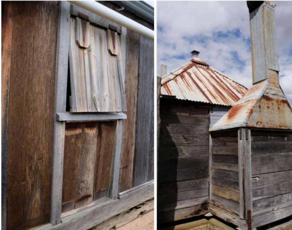
Figure 18. Left: Detail of reconstructed timber window awnings fitted to window openings on the north-west elevation. Right: View of the rear of the detached kitchen showing the roof, fireplace, and galvanised metal-clad chimney.
