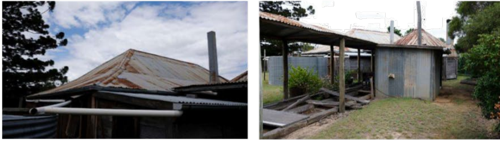
Figure 13. Left: The broken-back, hipped roof clad in corrugated galvanised iron of the main homestead building, with the roof of a small skillion structure also visible. Right: The covered walkway constructed of a post-and-sapling frame with a corrugated iron roof, with access to the galvanised iron-clad utilities area attached.
