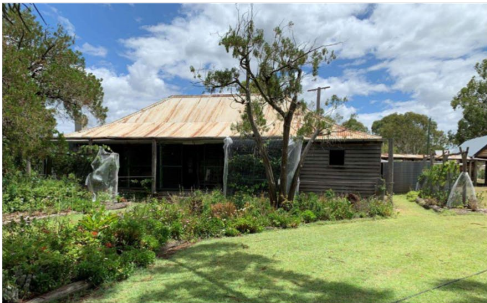
Figure 10. View of the front (north-east) elevation of the homestead. Note the established garden beds and its garden setting.
