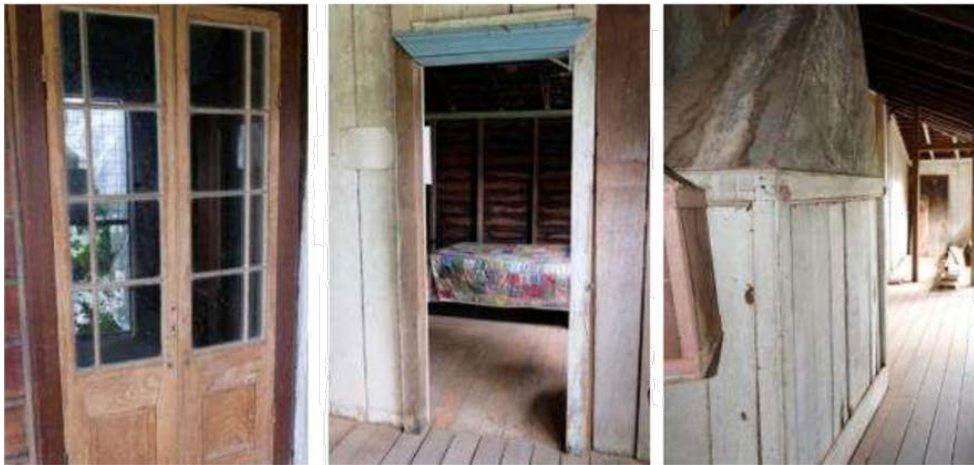
Figure 15. Left: The French doors on front verandah showing the reconstructed timber walls. Centre: View from front verandah to the north to the enclosed verandah sleeping area. Right: View along rear verandah to back of the fireplace.
