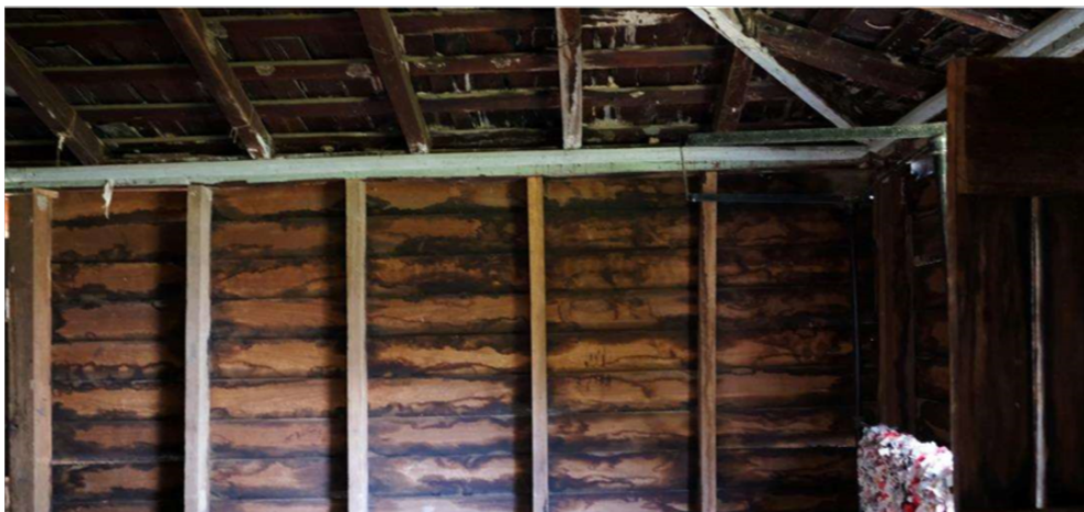
Figure 24. An example of the exposed single skin construction in the northern Bedroom 3 located at the enclosed verandah.
