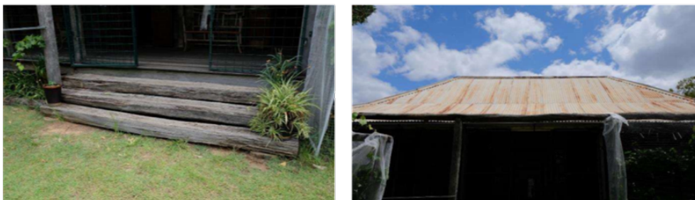
Figure 12. Left: The timber steps providing access to the front verandah of the homestead. Right: View of the front elevation showing the hipped roof clad in corrugated galvanised iron.
