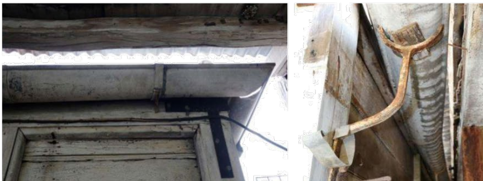
Figure 16. Left: Detail of the half round gutters surviving at the north wall of the kitchen. Right: Detail of a surviving bespoke metal gutter support at the junction of the kitchen and rear verandah.
