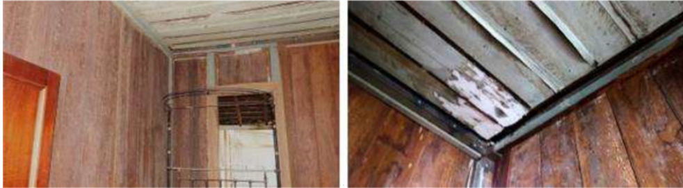
Figure 23. Left and Right: Interior views of Bedroom 2, noting water penetration affecting the ceiling, canvas linings are falling away, and movement at wall and ceiling junction.
