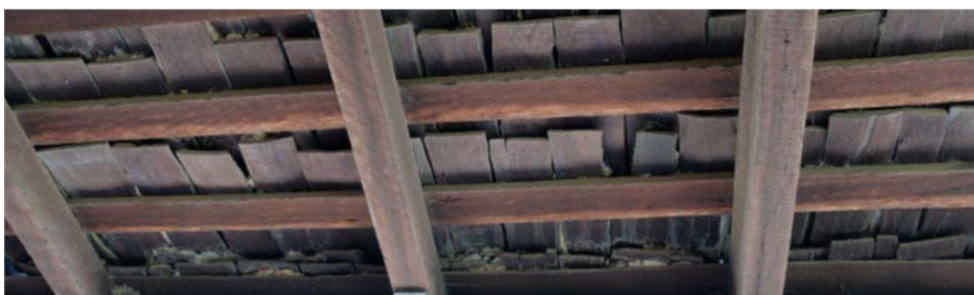
Figure 17. The underside of a section of the front verandah roof, showing the early timber shingles.
