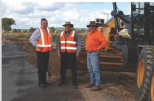
Mayor Kratzmann, Jeff Stephan and Lloyd Jorgensen inspecting the restoration work on River Road, Kingaroy
