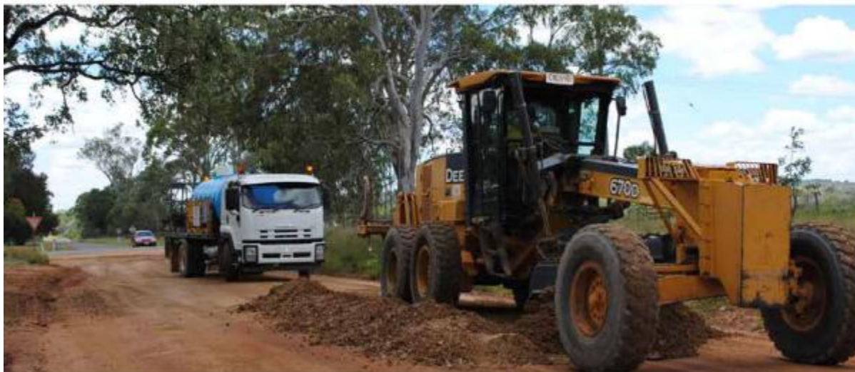
Flood Damage from the 2013 Floods
